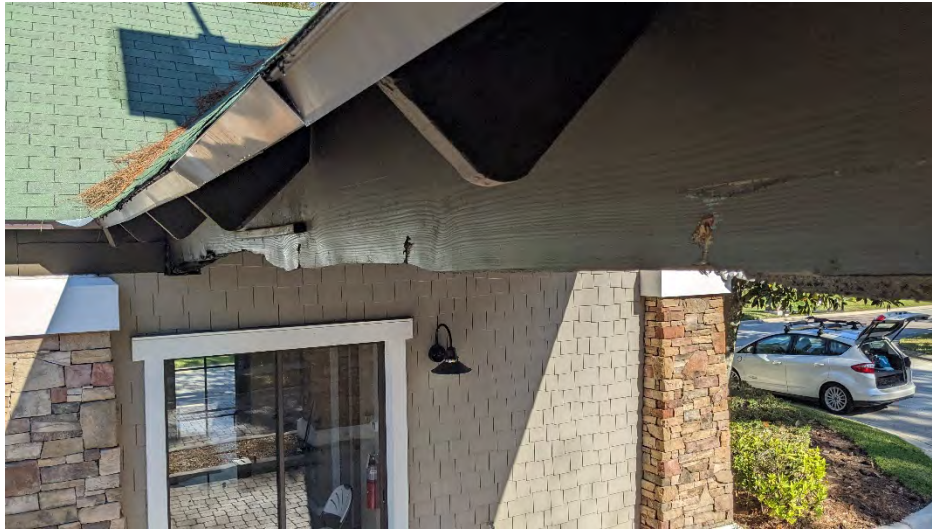
Photograph No.5 – Damaged wood beam at the exterior surface
